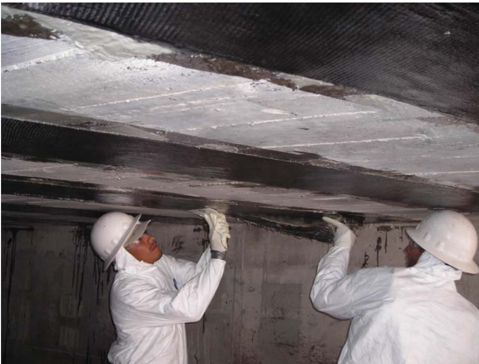
Application of CFRP fabric strips at the soffit on the 19th Avenue Bridge.
